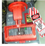
Circuit Breaker Lockout
