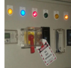
Electrical Panel Lockout
